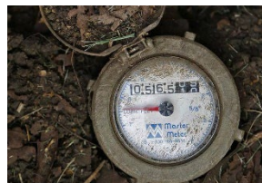
Customer meter under registration
